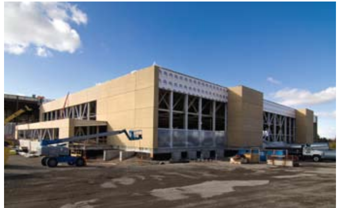
Work on the walls of the Auditorium multi-purpose area are near completion.
