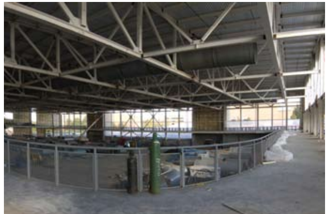
A suspended track has been put in place inside the multi-purpose area.
